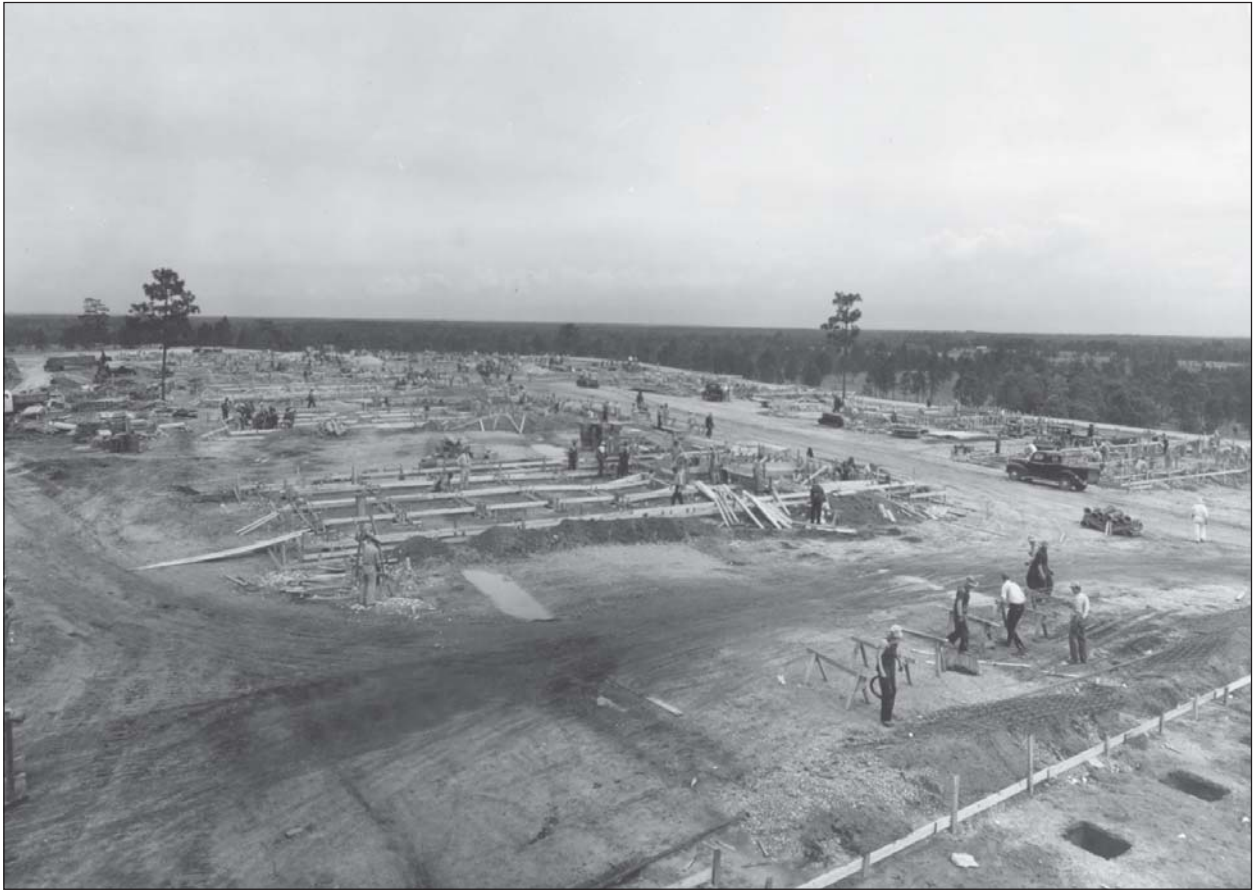
Workers lay foundations for Camp Polk buildings, June 12, 1941. Thousands flocked to Camp Polk for construction jobs.
