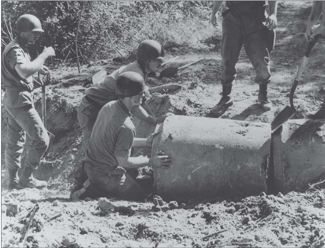
Fort Polk, long a training site for military engineers, housed the 588th Engineer Battalion, seen here installing a culvert in 1978.
