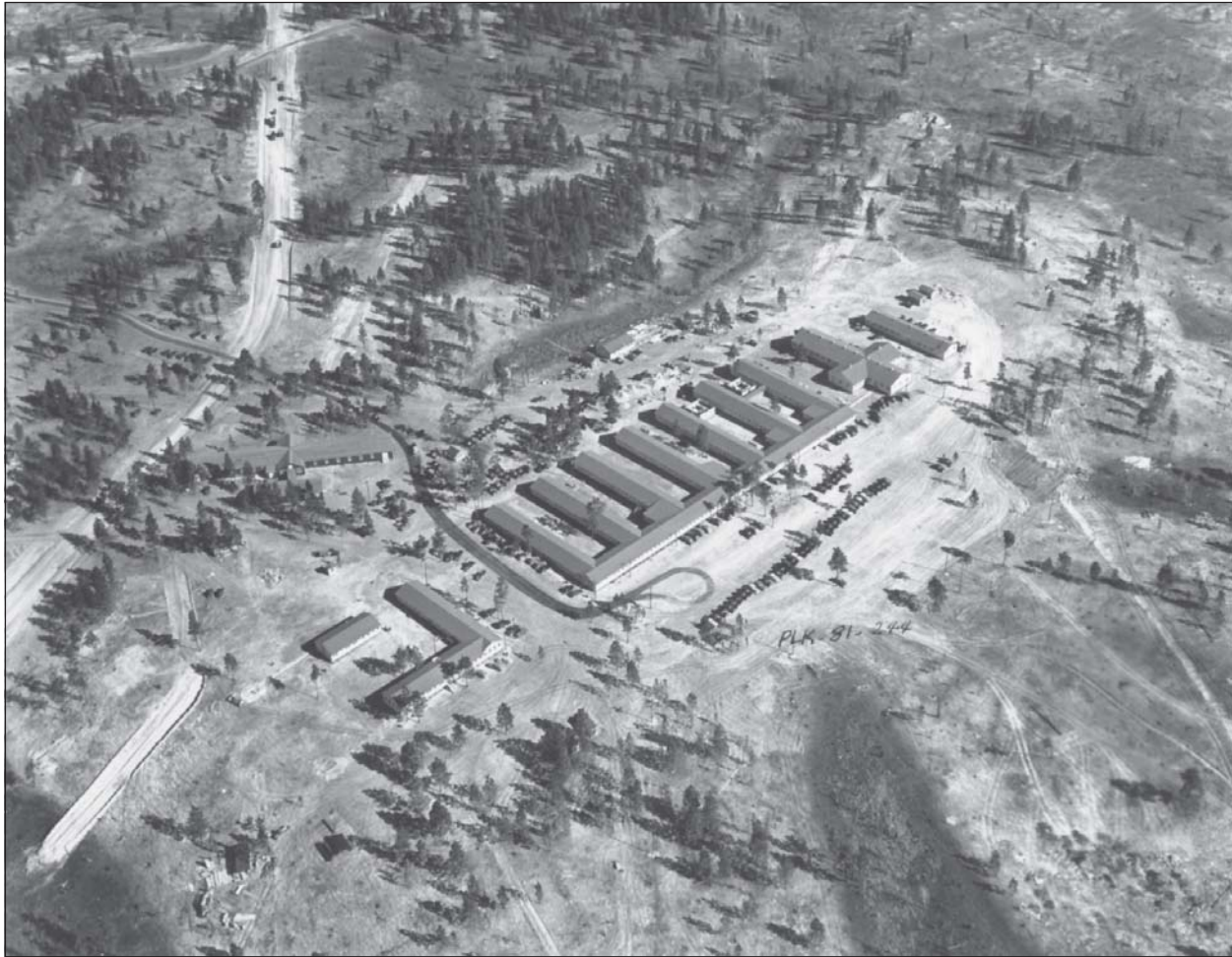
Aerial view of new temporary buildings in the early days of Camp Polk construction, February 2, 1941.
